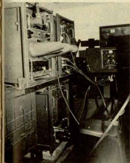
Interior view of the converted AN/TPS-1D showing Indicator, Modulator and Receiver Transmitter.
